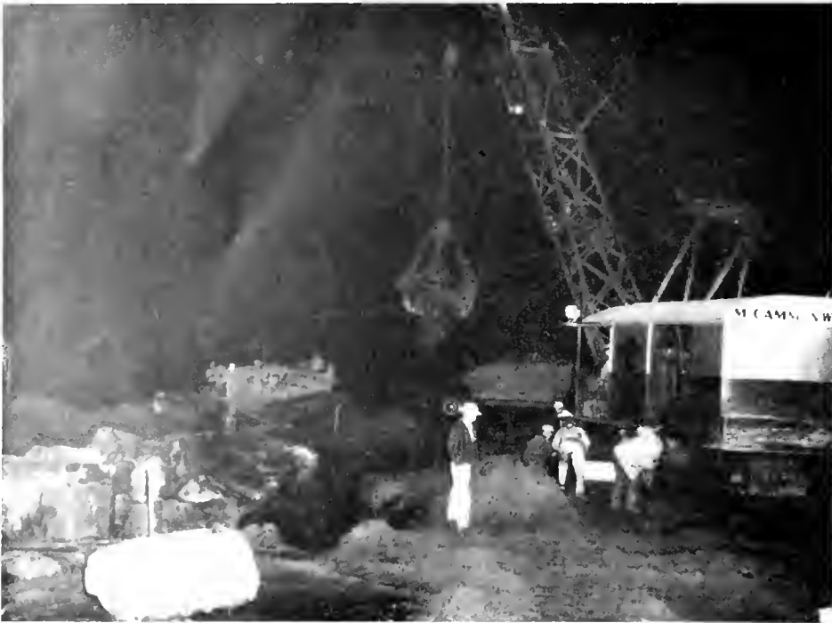
Limo 803 crane with 70-foot and 2-cubic-yard Esco orange-peel bucket with rock hooks placing rock backing in riprap section
